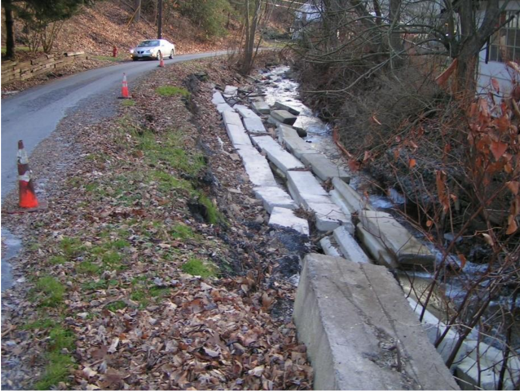
Figure 20 - Hurricane Lee September 2011 – Brewery Run Road After
