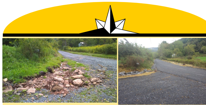
Before After Beech Creek Twp. Falls Road Dirt & Gravel Roads project. Road fill used to reshape and crown road so stormwater leaves the roadway and flows to buffer along stream or into armored ditch with underdrain. Spring water captured with 250' underdrain and reconnected to the stream. Over 650' of road surface stabilized.
