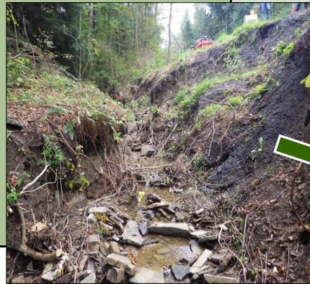
BEFORE – Picture above taken from Selfe Rd in Bald Eagle Township. The Road shoulder and streambank were collapsing with direct sedimentation to a tributary to Sugar Run.
