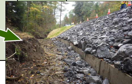
AFTER – Streambank stabilized decreasing the chance for road failure and sedimentation to stream.
