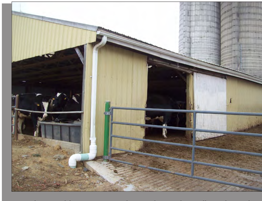
A roof gutter and downspout connected to an underground pipe collect and carry clean water away from this animal concentration area.
