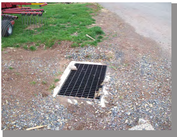
This surface inlet carries runoff and prevents scour along the existing driveway to the right.
