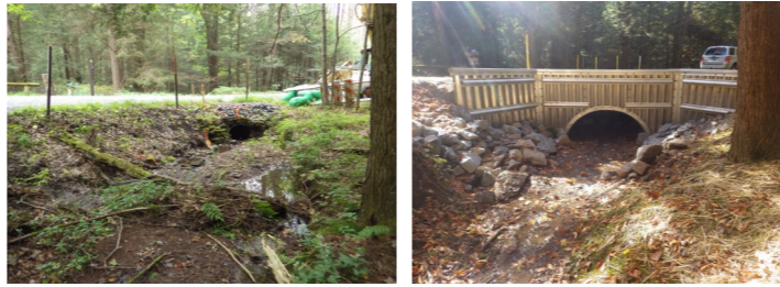
Pictured above is a stream crossing on Harbaugh Road in Greene Twp. before and after a culvert replacement project. The culvert pipe was undersized and impacted the road and the stream by causing erosion, not passing high flows, and being a barrier for wild trout in a Class A trout stream. Greene Twp. utilized the CCCD's Dirt, Gravel and Low Volume Road Program Funds to install a proper culvert to solve the stream and road problems.
